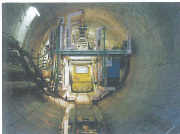
Fig. 2 10 meters of tunnel will be excavated per day using the shield tunneling method. Anchor channels and grounding connections are already mounted in the precast concrete plant of Max Bögl.
